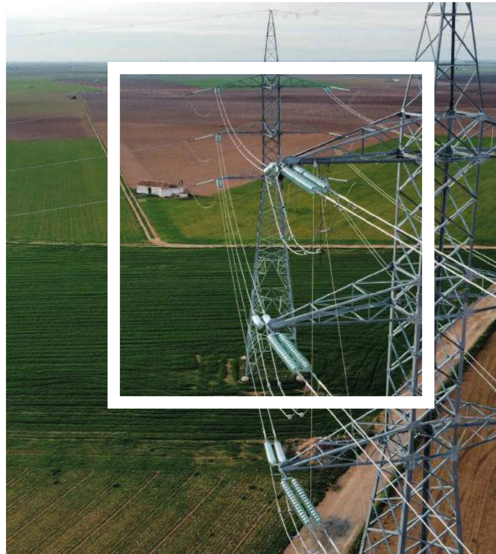
Insulator replacement on the evacuation line of the Nudo Manzanares SET (Spain)
