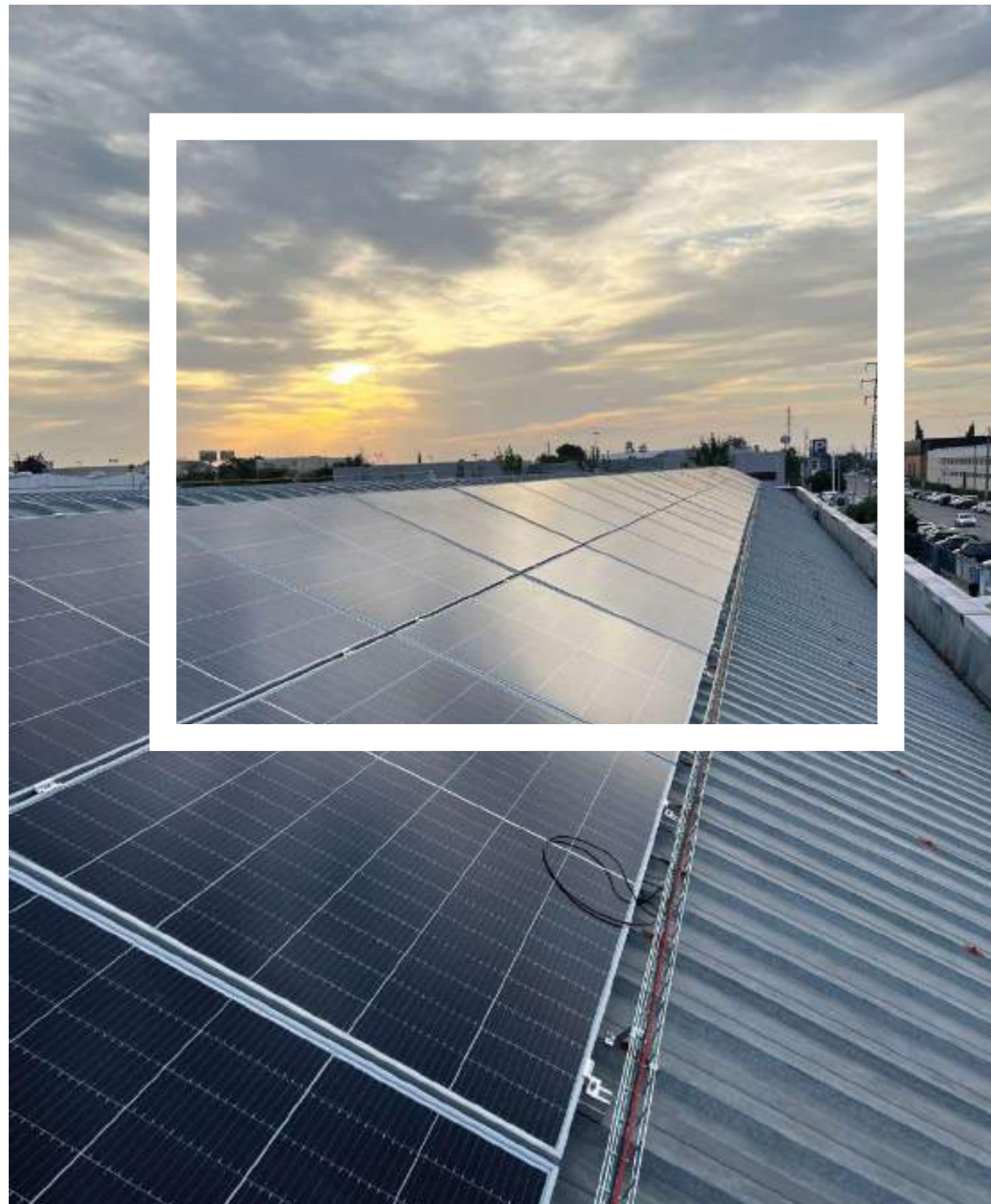
Warehouse photovoltaic facilities for self-consumption in Getafe, Madrid (Spain)
