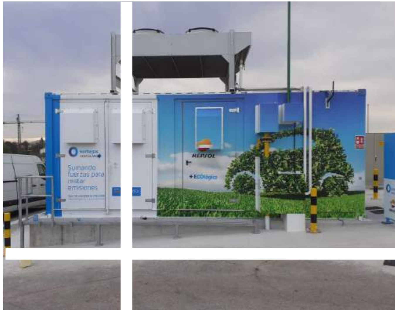
Compressed gas refuelling station for vehicles, Cantabria (Spain)
