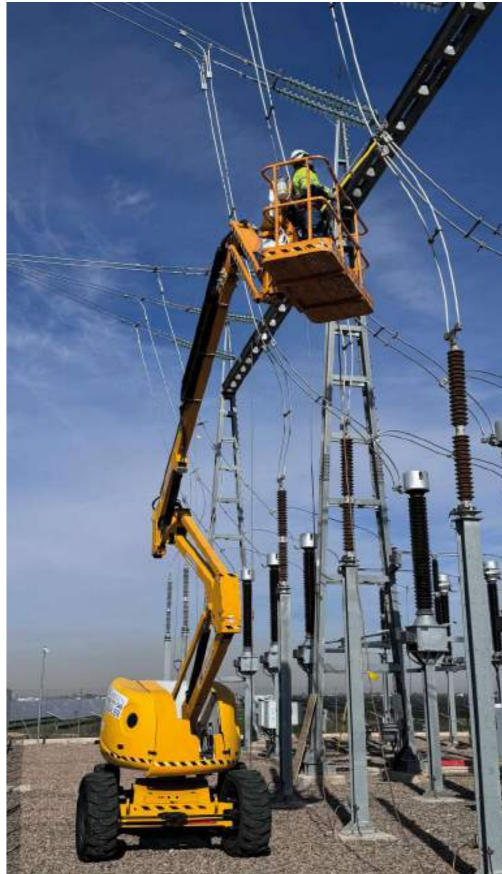
Insulator replacement on evacuation line at the Nudo Manzanares Transformer Substation (Spain)
