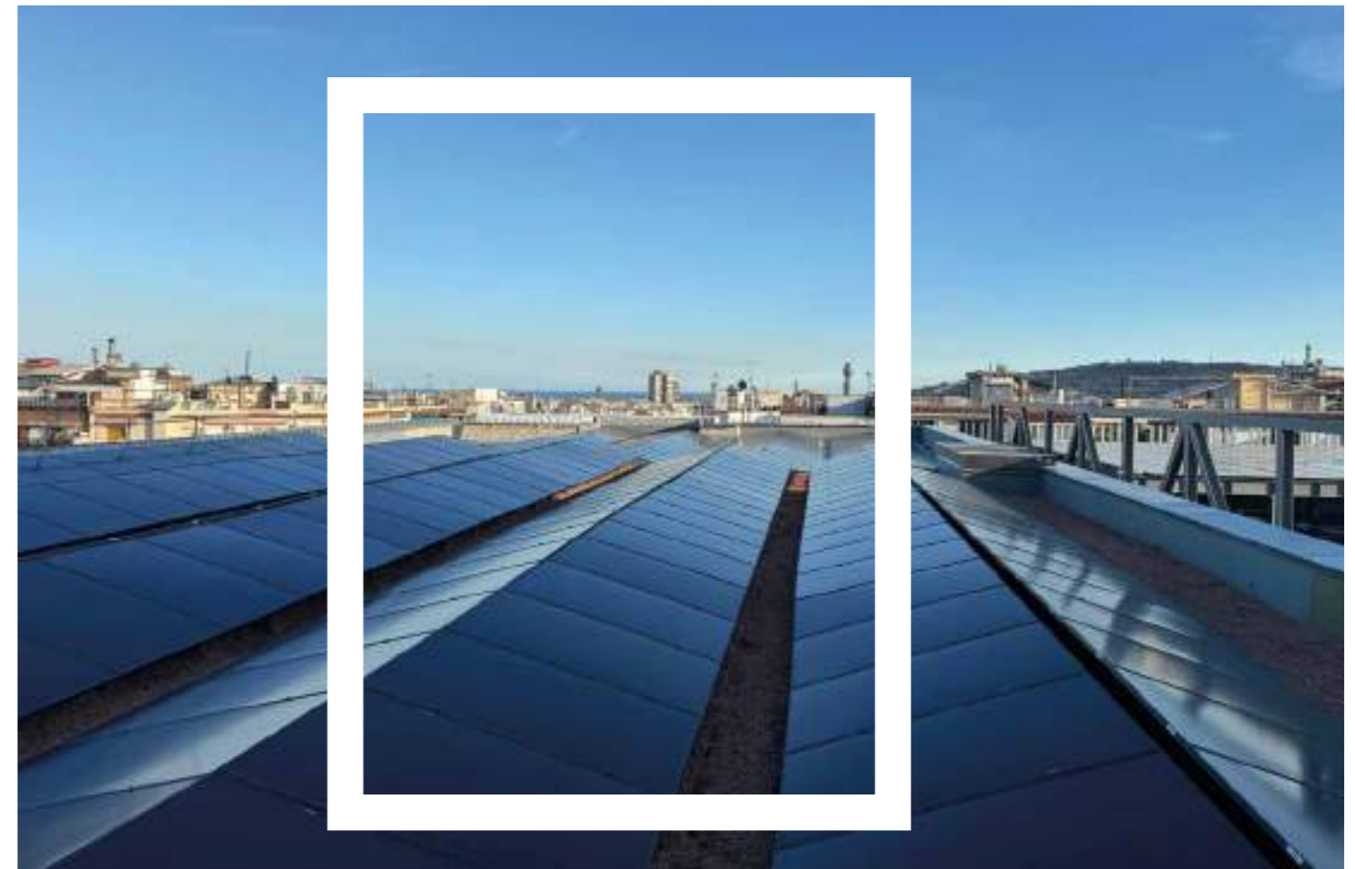
Refurbishment and restructuring of the building for El Corte Inglés on Diagonal into offices and commercial premises, Barcelona (Spain)
