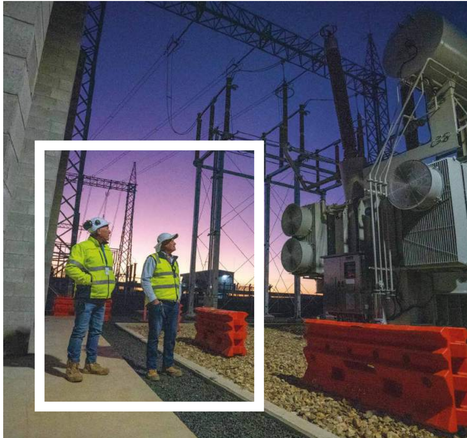
Substation of the New England Solar PV Plant (Australia)
