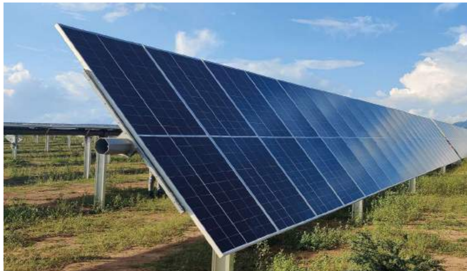
Esperanza solar photovoltaic power plant (Dominican Republic)
