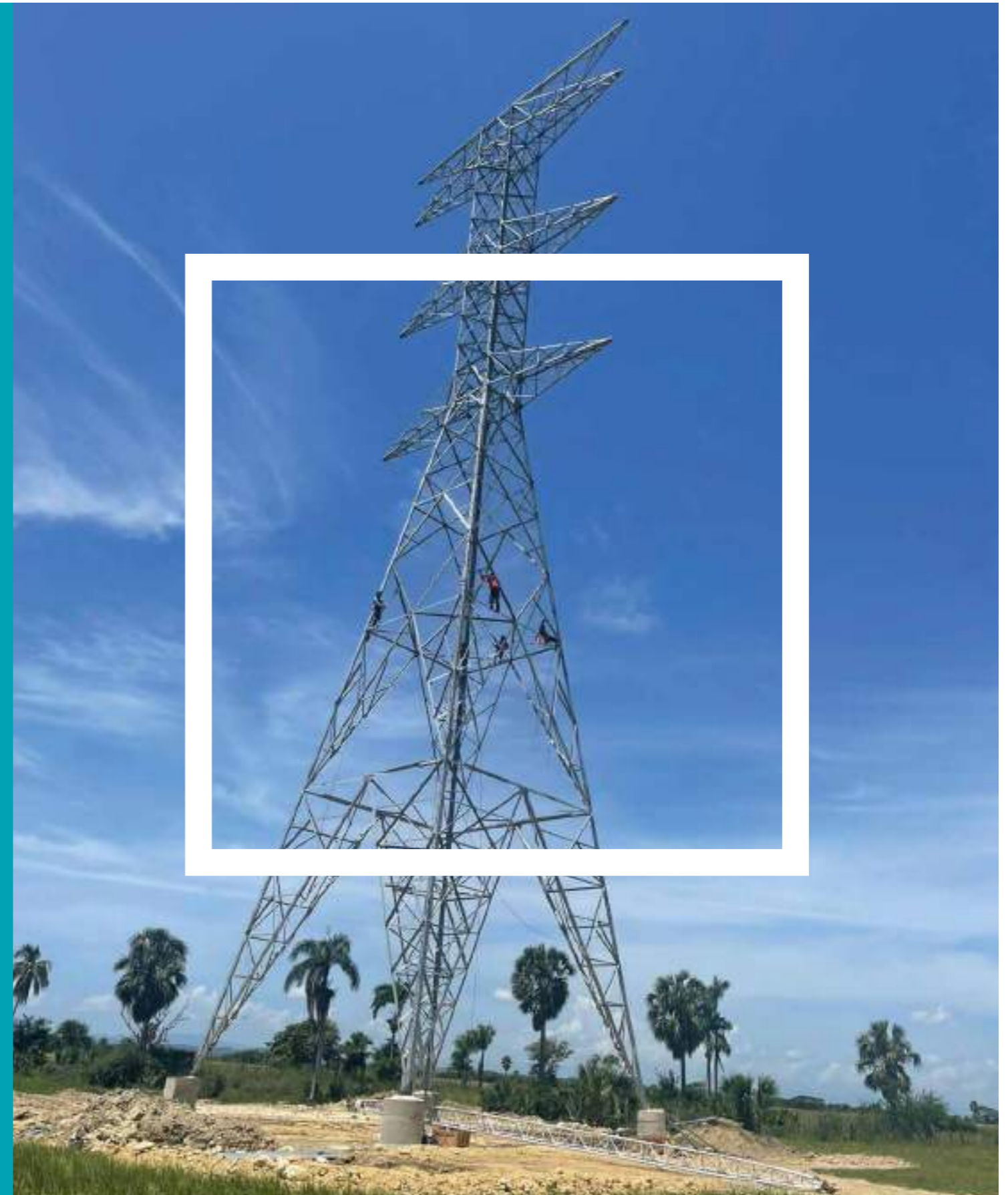
Guayubin-Manzanillo line (Dominican Republic)
