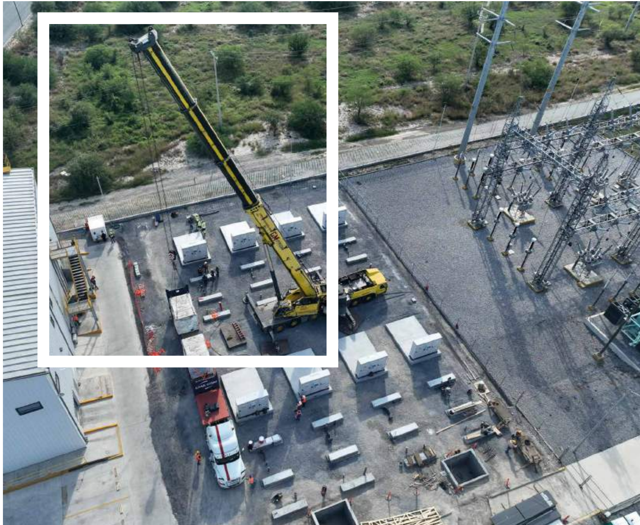
Storage with BESS batteries in Monterrey (Mexico)
