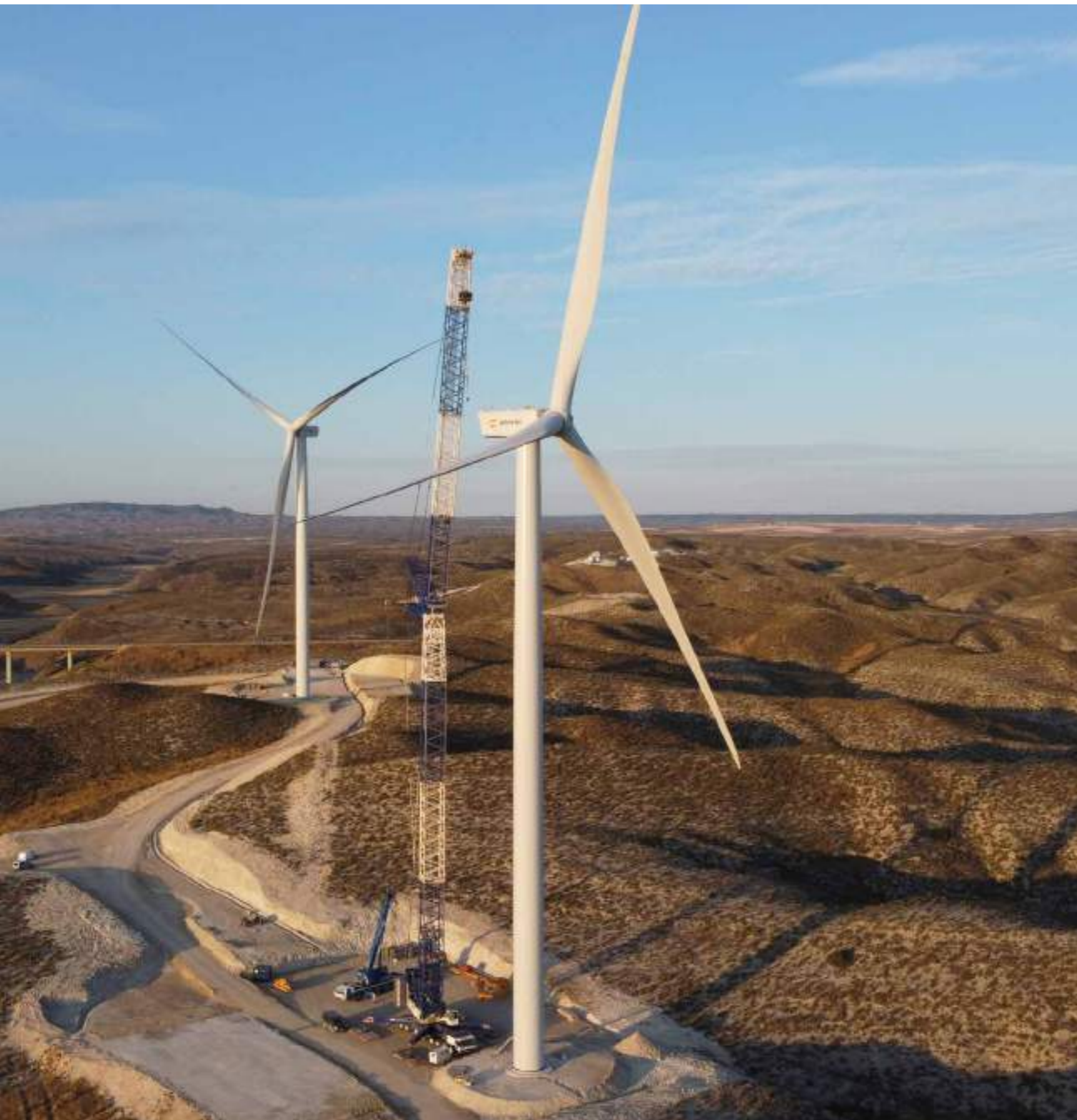
Monlora Wind Power Complex, Zaragoza (Spain)
