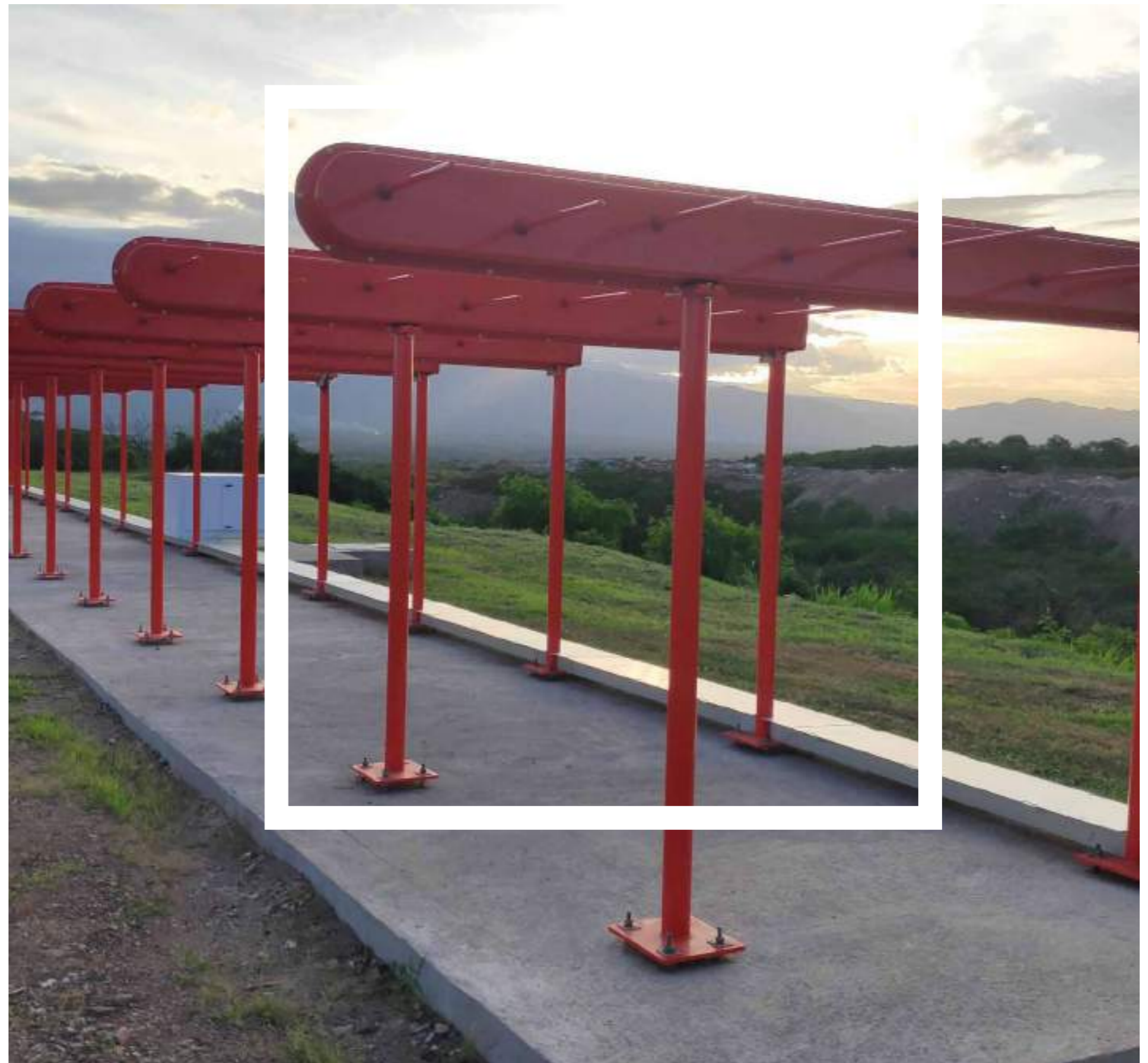
ADS-B system at the Palmerola Airport (Honduras)
