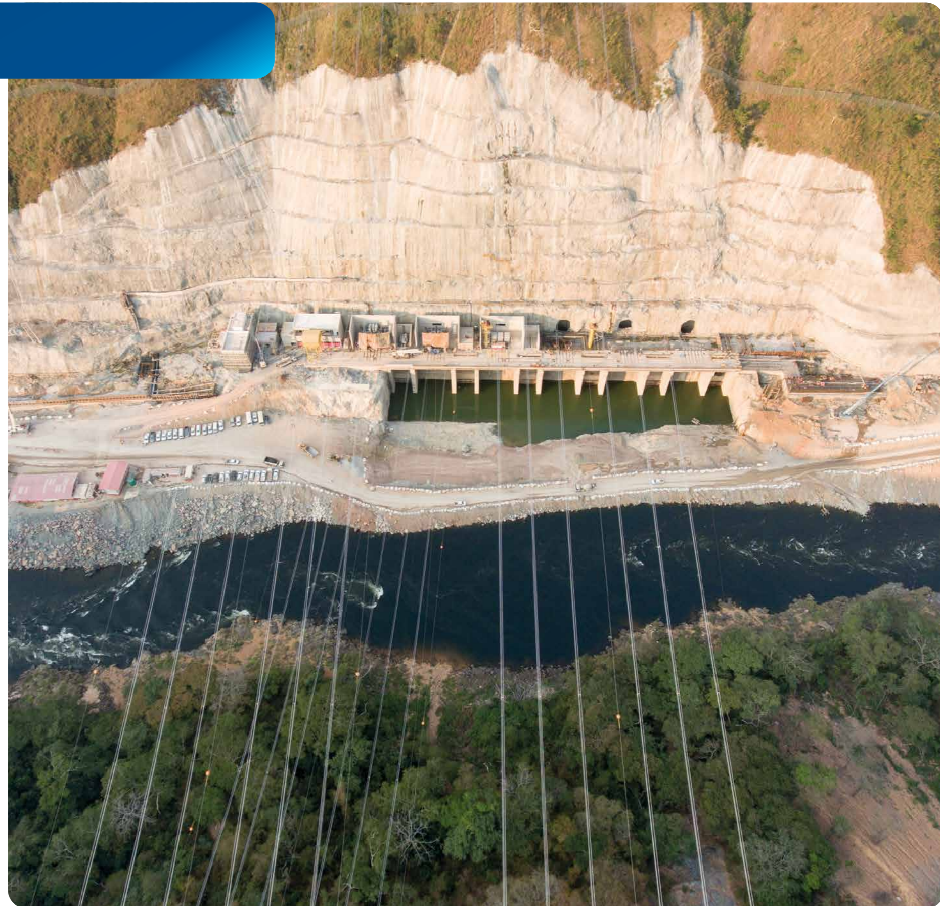
Laúca hydroelectric plant (Angola)
