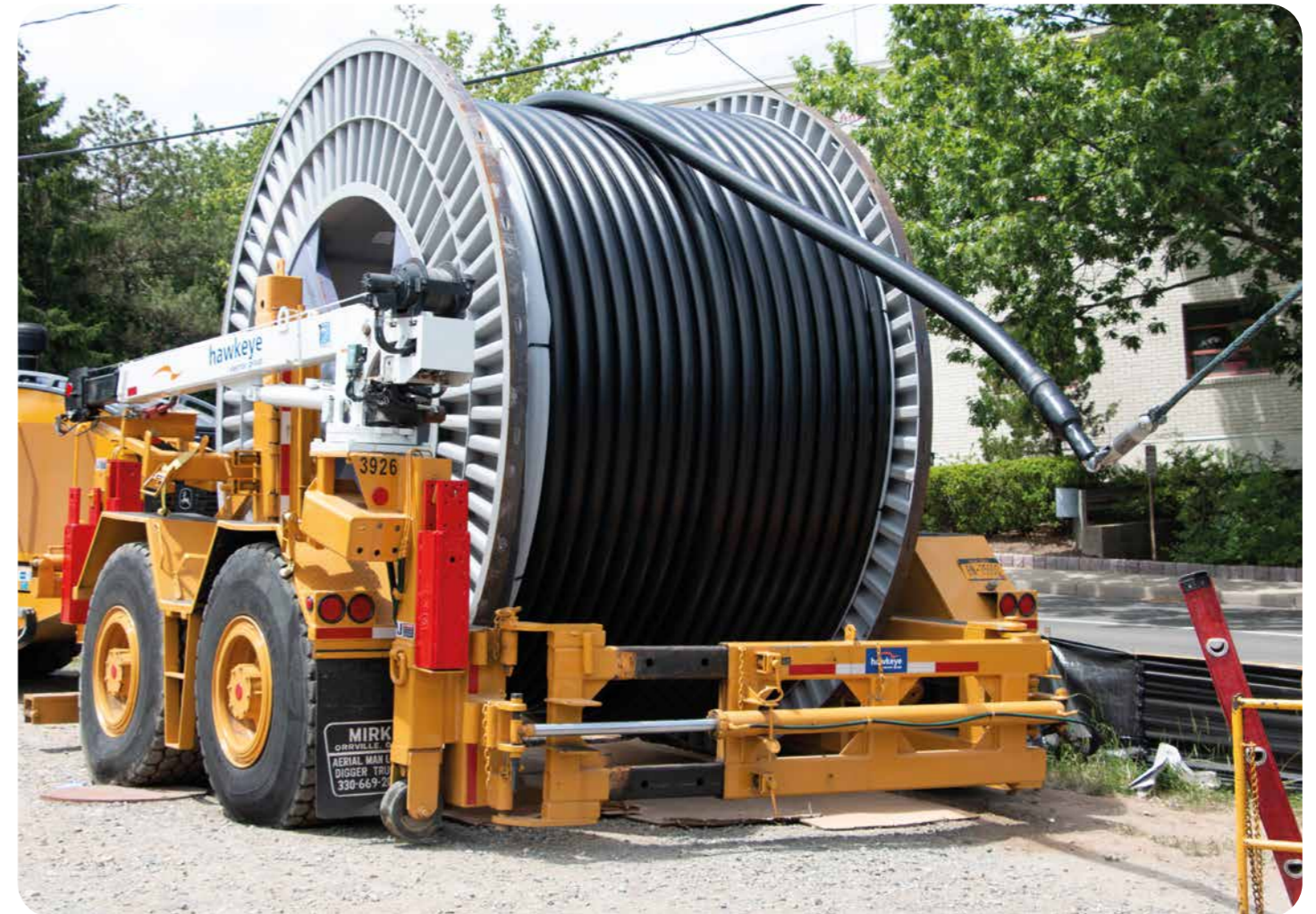
Underground power transmission line (United States) Hawkeye
