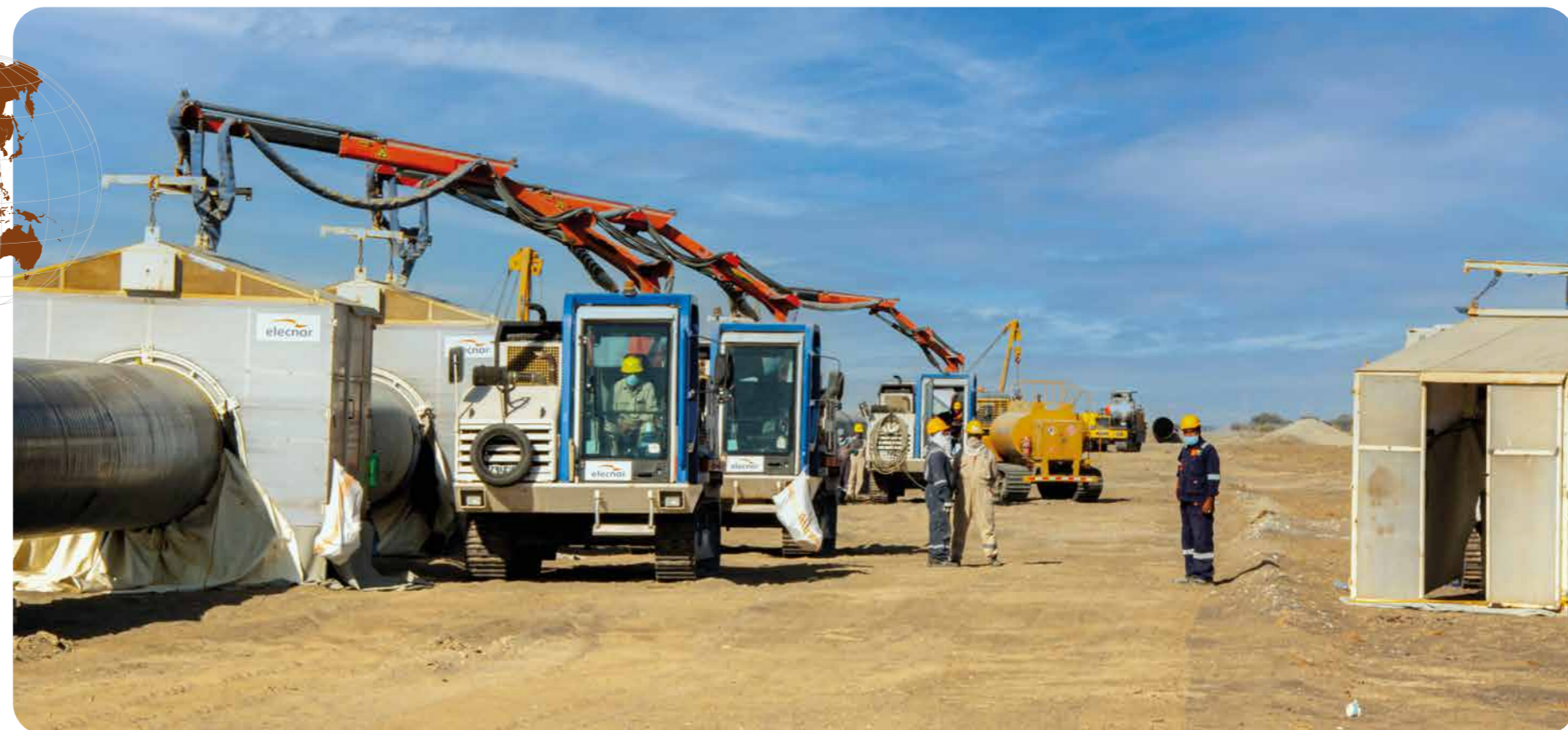
Water distribution network in Al Batinah (Oman)
