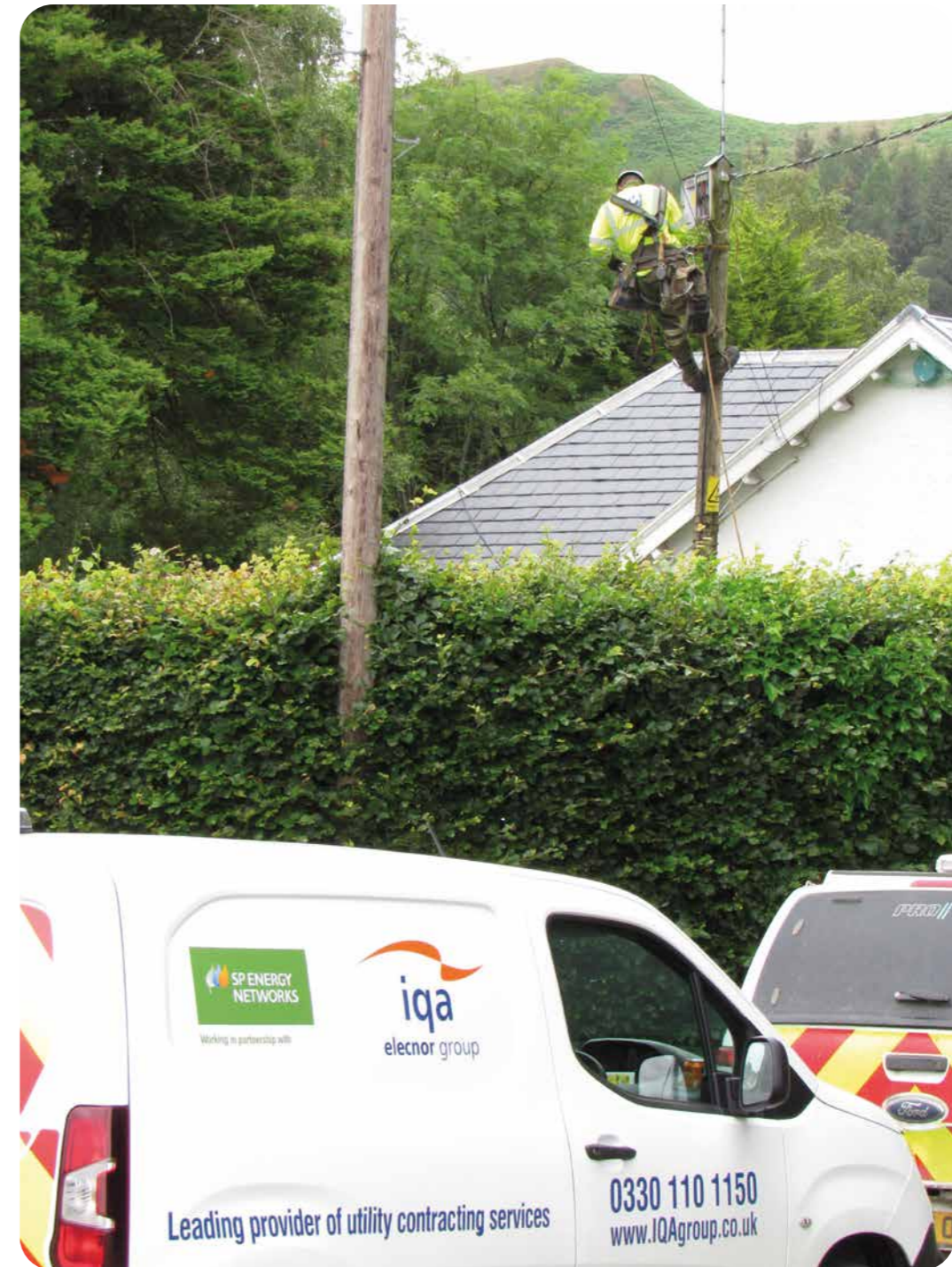
Overhead distribution line in Glasgow (United Kingdom), IQA
