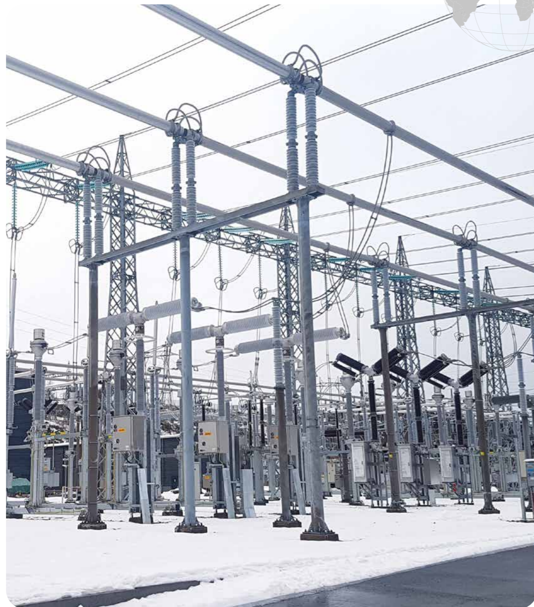
Kristiansand substation (Norway)
