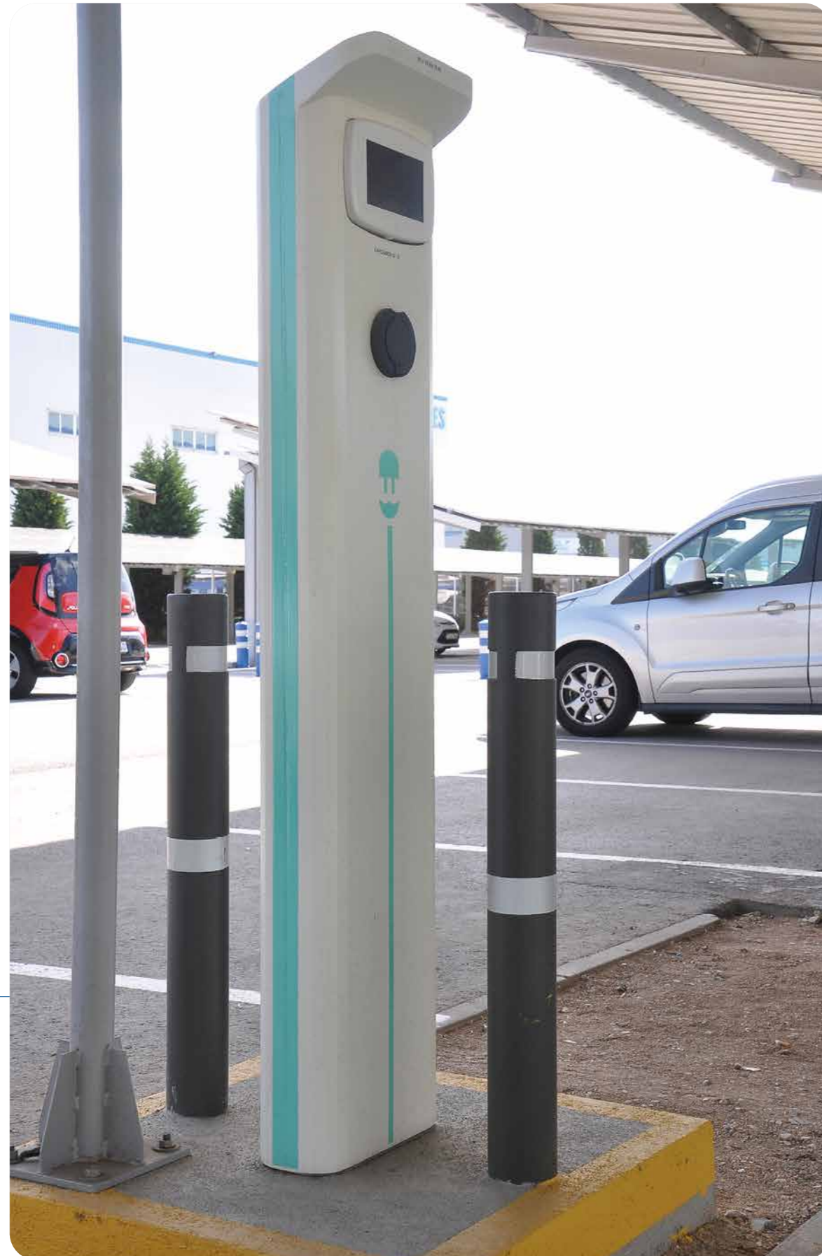
Electric vehicle chargers in Barcelona (Spain)
