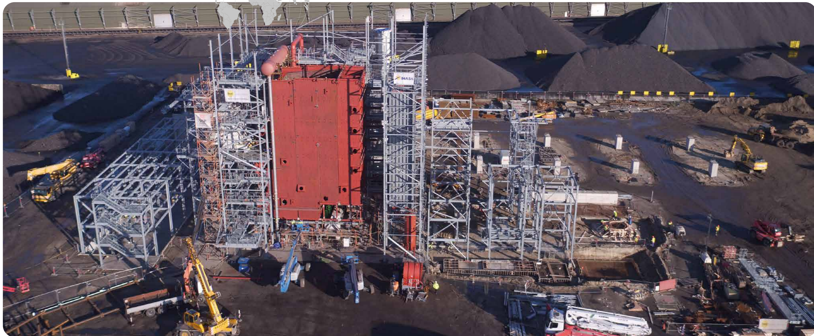
Biomass plant in Gante (Belgium)
